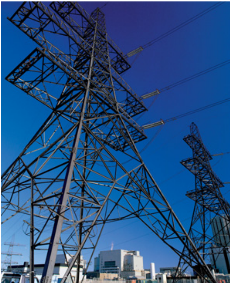
BNG profits from commercial power stations but will refocus on decommissioning. Photo courtesy BNFL
