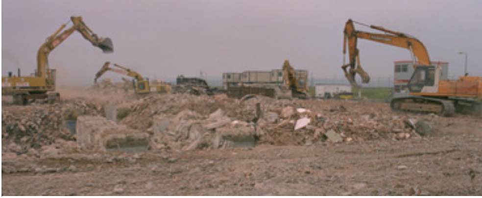
Demolition could be a part of decommissioning where privatisation can drive down costs. Photo courtesy BNFL
